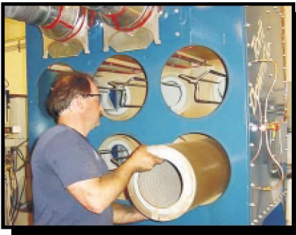
Image 2 - Filters installed on Dust Collector
