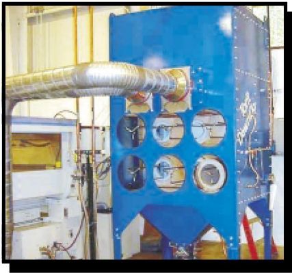
Image 1 - Full view of Dust Collector
