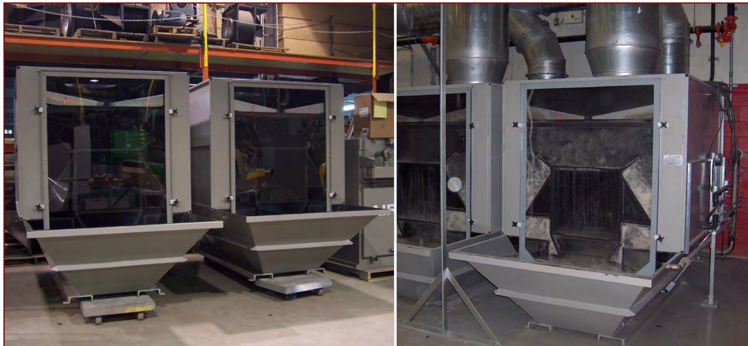
Aluminum buffing/grinding - ducted system Aerospace
